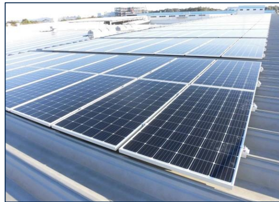
Ashimori Industry Yamaguchi Co., Ltd. Solar Power Generation
