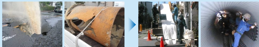
Increasing number of aging pipelines
