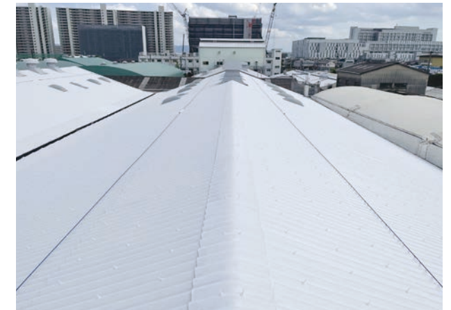
Heat-shielding paint on the roof of the Head Office and Osaka Plant
